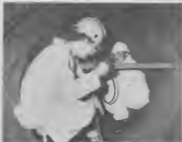
D.P. Mendez and F.A. Sota using a boroscope to inspect the internal condition of tubes in a waste heat boiler at SIAR.
